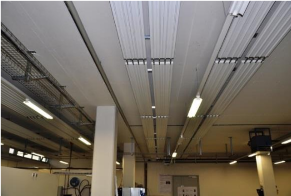
Cold ceilings (Zehnder) installed in the Lab.
