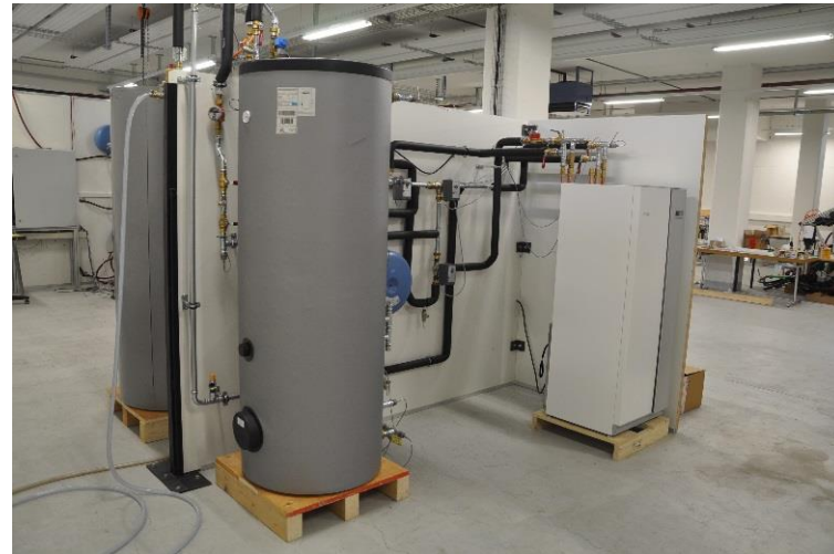
Cooling machine (HP; ait / Nibe) & storage tanks.
