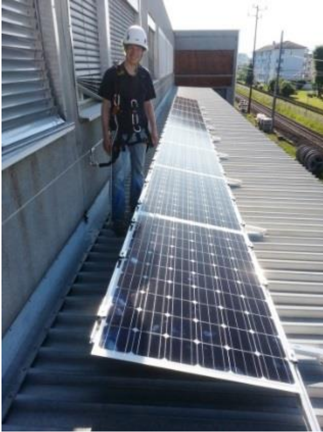
PV modules (Meyer Burger) – south oriented
